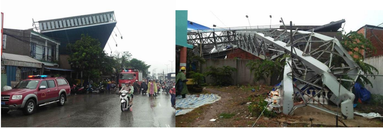
Figure 2. Damage of Billboard and partial damage building (Highway 1A, Binh Tan distric, Ho Chi Minh city, 10 August 2018) [7]
