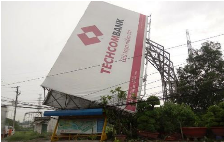
Figure 3. Damage of Billboard and partial damage building (Dong An industrial area, Binh Duong province, 7 August 2013) [8]
