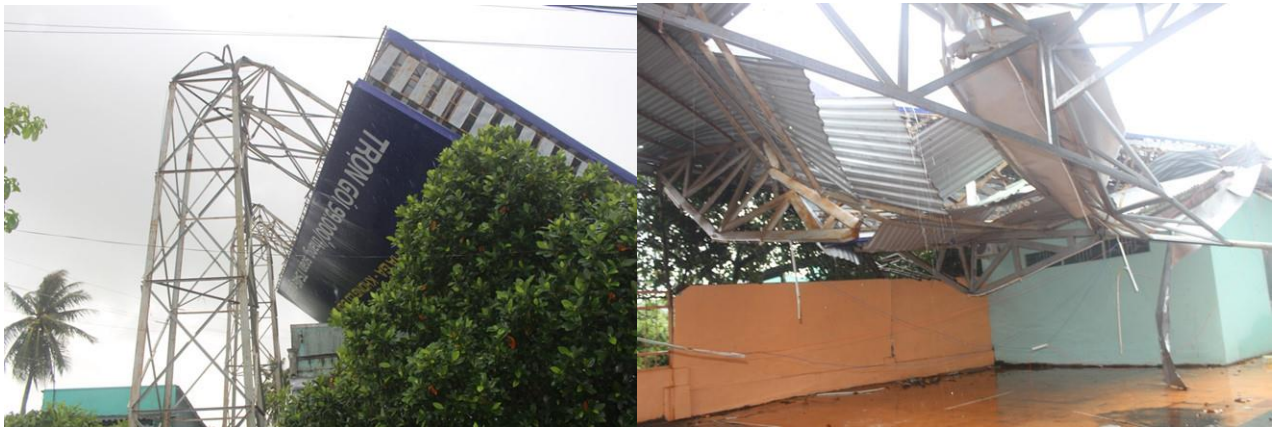
Figure 1. Damage of Billboard and partial damage building (Highway 1, Bac Lieu province, 3 August 2019) [2]
