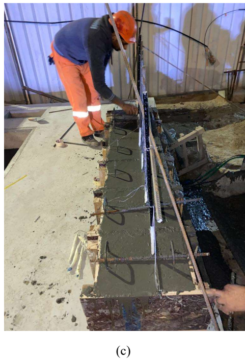
Fig. 4 —(a) expandable cement grout used for anchoring steel tubes to GFRP bars; (b) Anchor setup used to cast the grout; (c) embedding the L-shaped GFRP bars after casting the concrete cubes.
